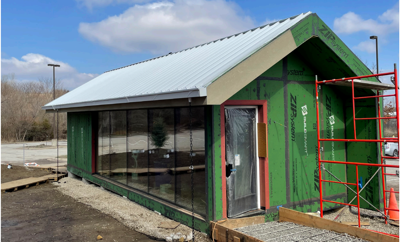
Haven Studio, photo showing the quad-pane windows supported by the steel frame made from reclaimed materials.
